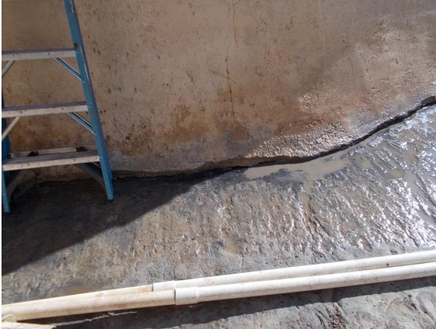
Fig 2: This photo shows how the gunnite has shrunken from the bedrock floor.
