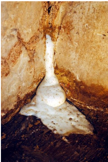
As HyperFlex reacts and fills the void, foam is visible at the injection site.
